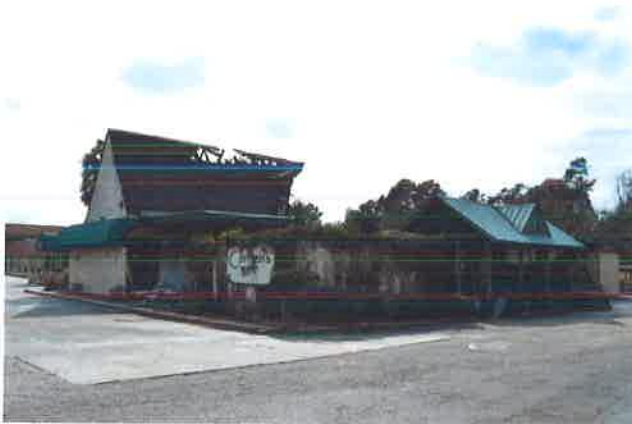
Adjacent partially burned down Carmen's Restaurant is located to the South of the Site.
