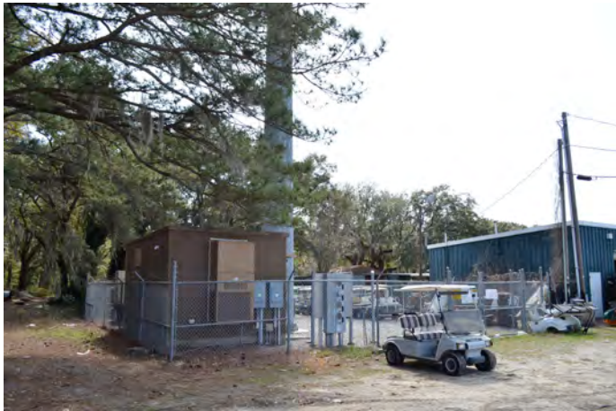
A cell phone tower is located at the Northwest corner of the Site on Sutcliffe Drive.
