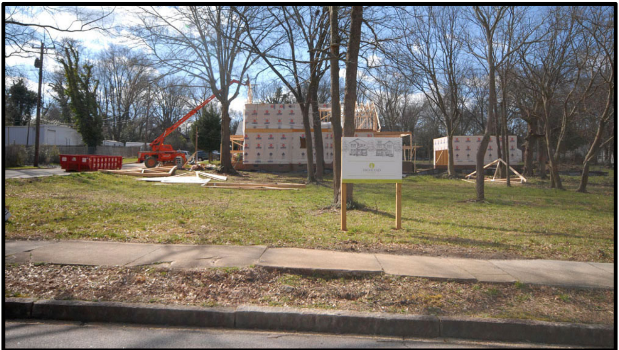
Photo 6—New homes being built on Stratham, two blocks from the site. Other homes in this neighborhood by the same developer are listed at $350k. See appendix.
